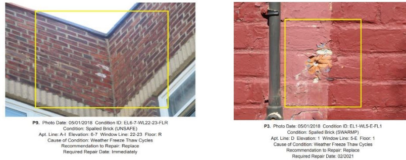
Figure 3: Pictures of building façade defects as shown in pages of façade inspection report
