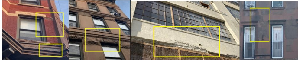
Figure 1: Residential buildings in Brooklyn with building façade defects
