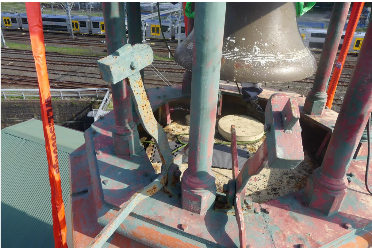
Figure 3. The base of the belfry, prior to removal. Note the clapper mechanism, and the circular cap was the maintenance access point. (Long Blackledge Architects 2014)
