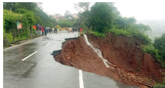
(Landslide dated on 29/09/2021)
